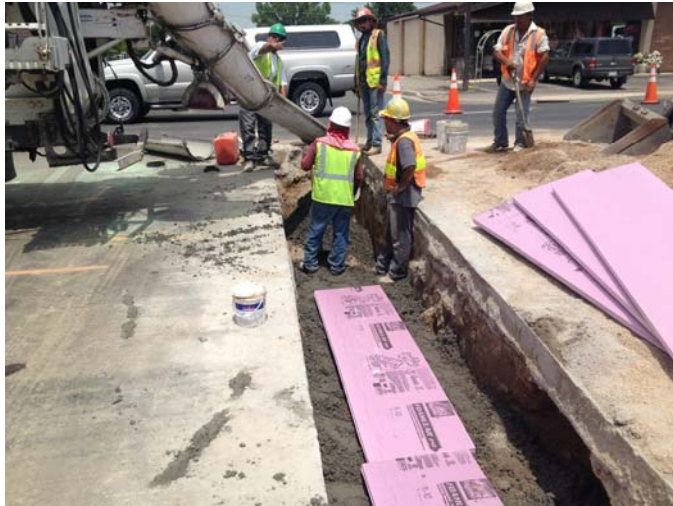
Sanitary Sewer Main for Lot 3 installed from 44 th Ave on Vance Street.
