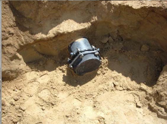
8" fire sprinkler line cut and capped 10 feet west of sprinkler valve pit.
