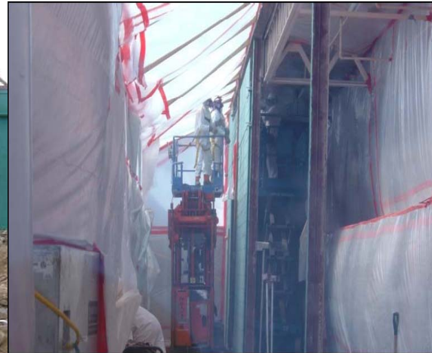
Abatement crews working on hand demolition removal of Antique Mall east exterior wall.
